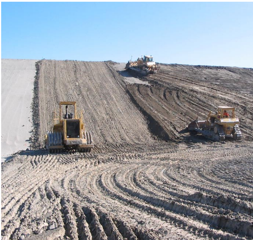
The Washington State Department of Ecology has issued a temporary authorization to allow installation of the earthen liner at the bottom of the Integrated Disposal Facility.
